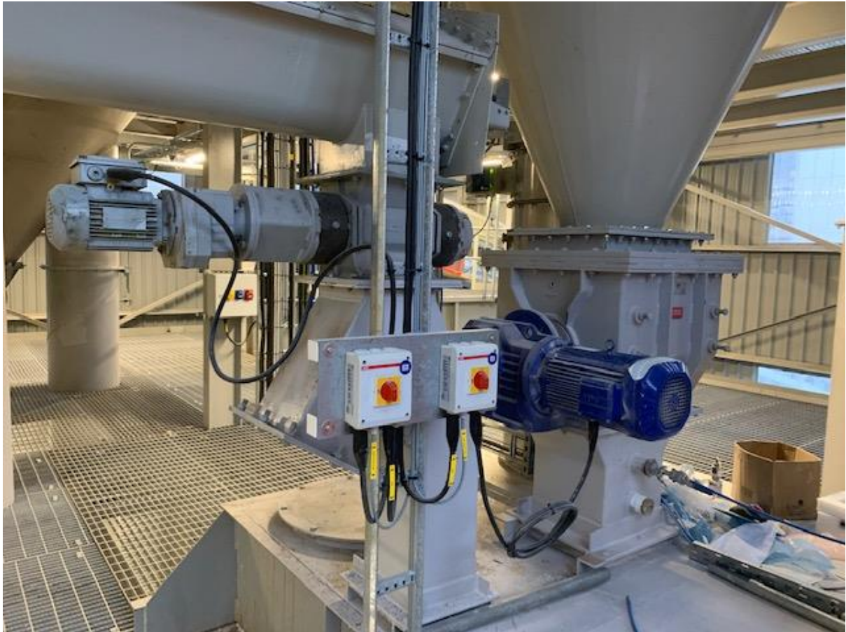
Cyclone and Filter Material combine in surge hopper with in-process particle sizing
