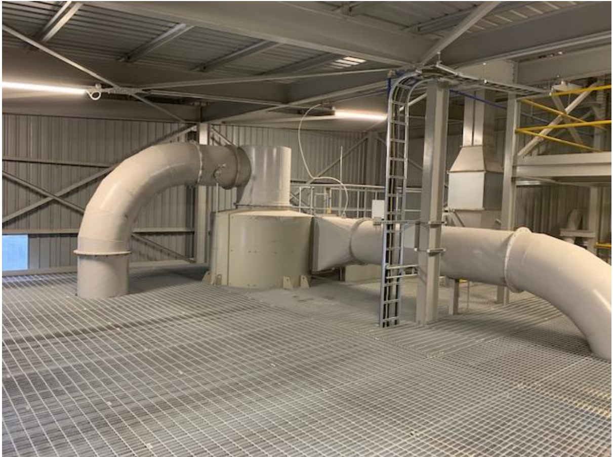
Cyclone Inlet and Air Discharge
