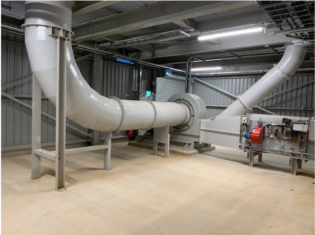
Main Fan and Two-Stage Modulating Burner providing efficient in-circuit drying
