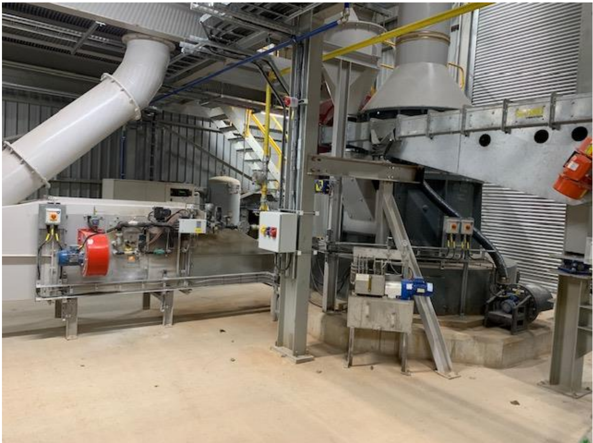
Burner and Mill Feed Arrangement
