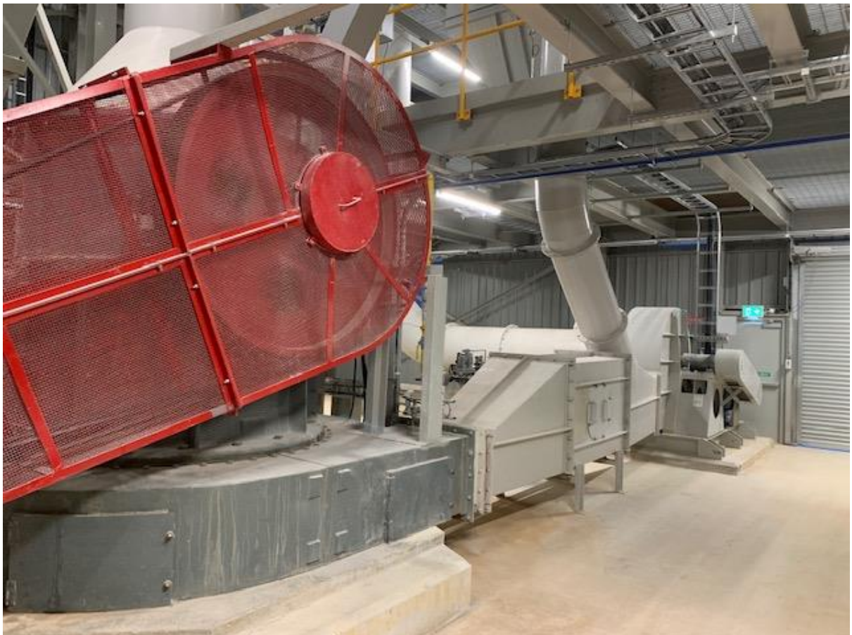
Air Inlet Ducting to Mill and Main Fan
