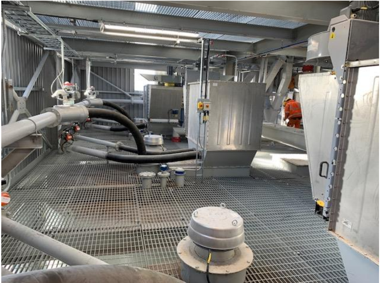
Powder Silo tops with diverters, filters, and instrumentation
