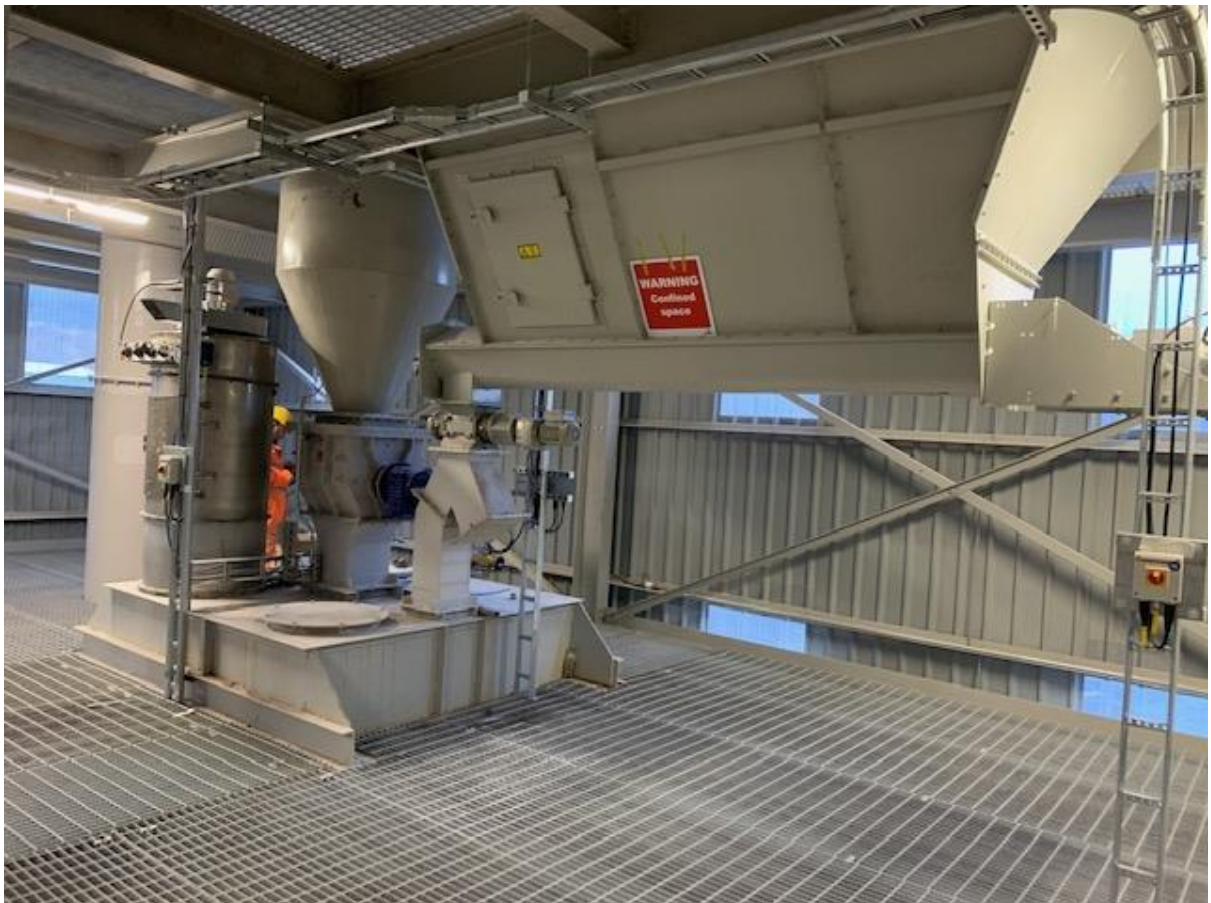
Vent Filter and Cyclone Discharge
